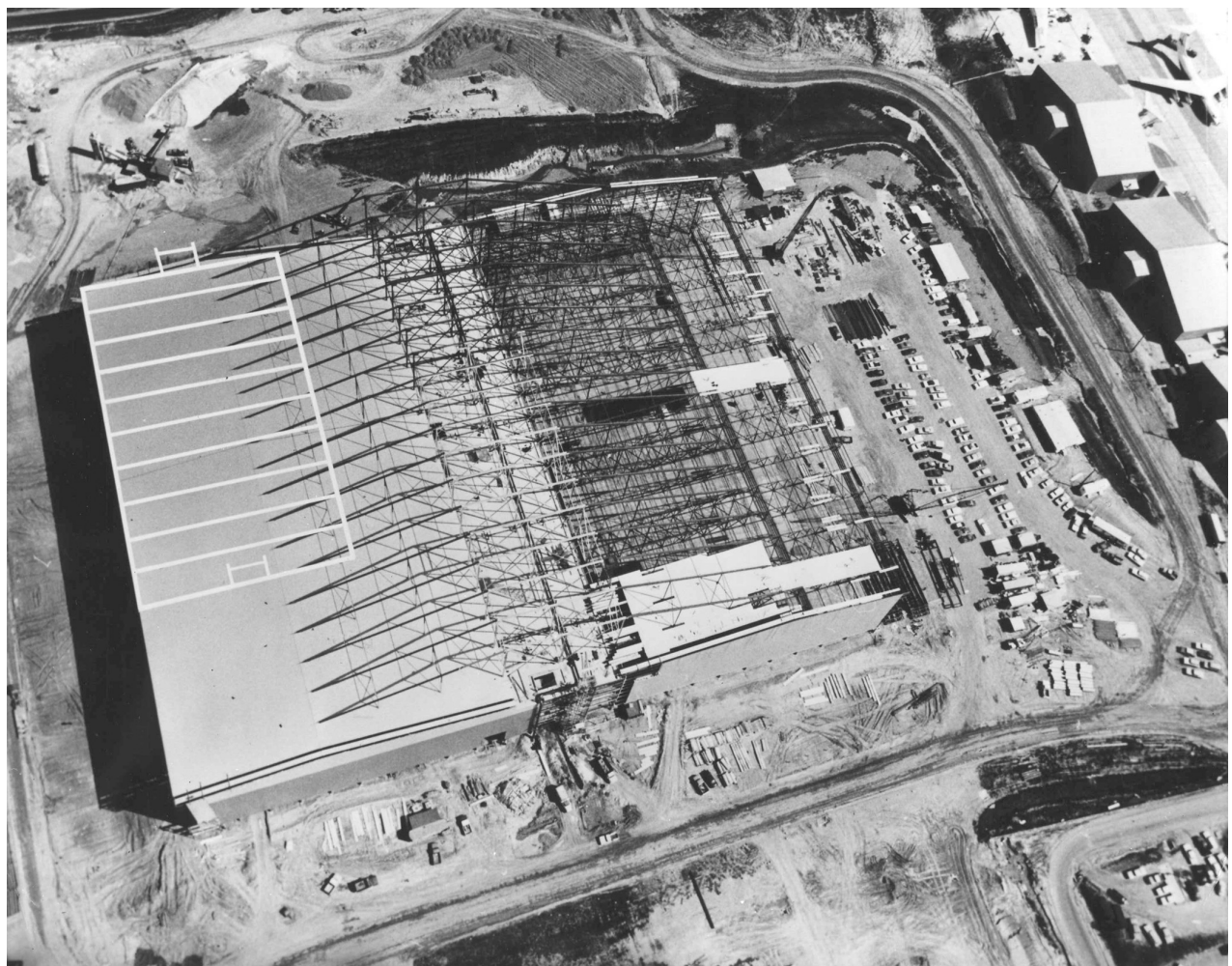
Aerial view of C-5A Test Center (L-10) under construction, May 1967. The building was believed to be the largest cantilevered hanger in the world. Note the scale model of a football field superimposed in the upper left corner.
